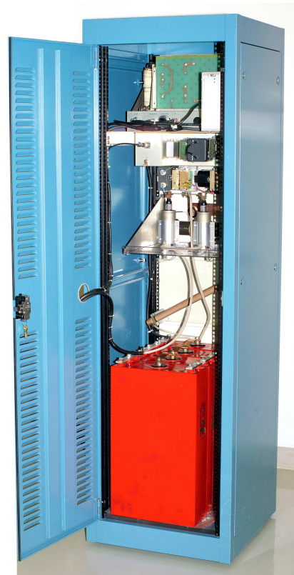
Figure 4. Photograph of 11.8 kJ bank, back of the cabinet.
