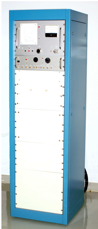
Figure 3. Photograph of 11.8 kJ bank, front of the cabinet.
